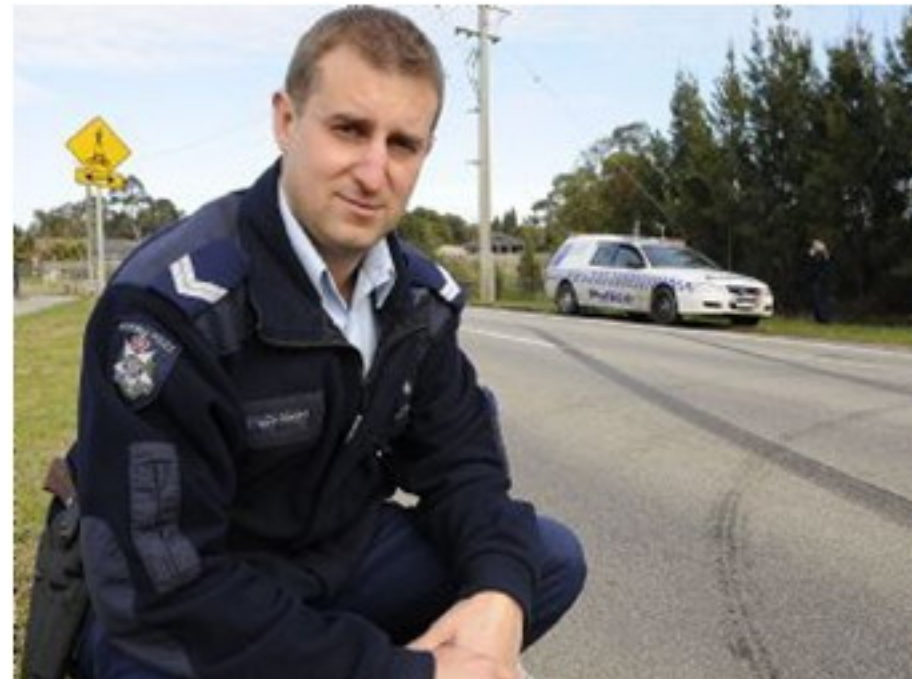
Senior Constable Chris Jolly from Rowville police with marks caused by hoons in Karoo Rd, Rowville. N04KN30
